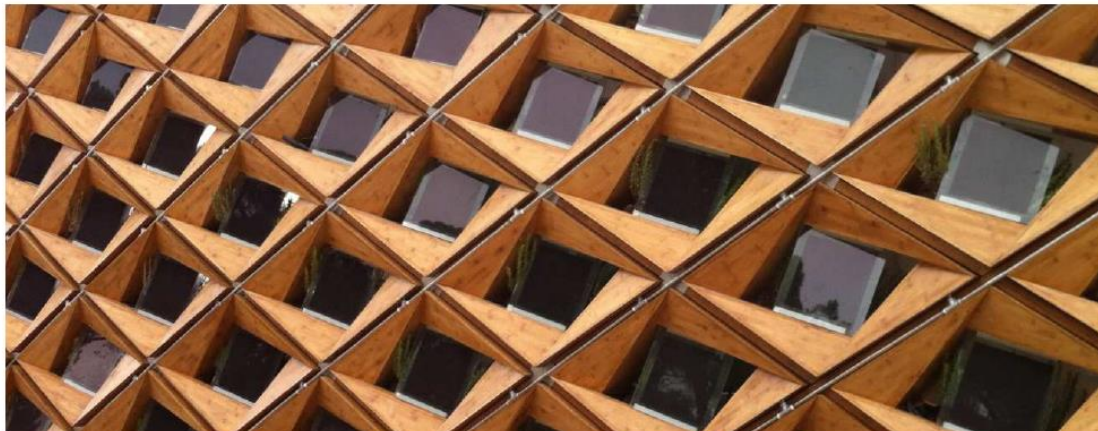
FIGURE 19: A COMPLEX BIPV FACADE IN THE SOLAR DECATHLON "PARA ECO HOUSE" (SOURCE: C. POLO, SUPSI)
